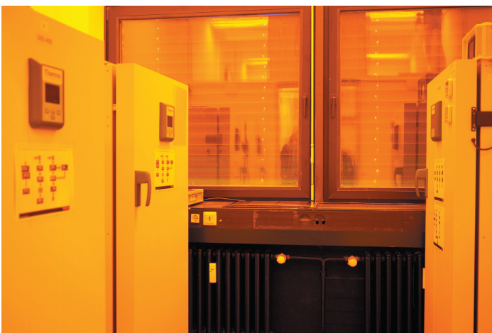
View of the heating cabinets
