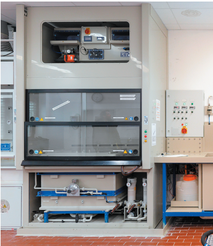
Etching unit with fume hood and exhaust air filter system
