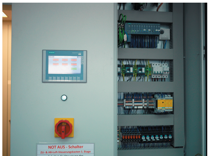
Controlling the air supply and exhaust air system
